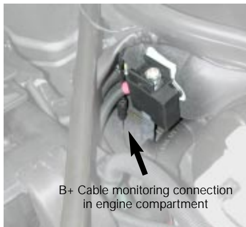
Battery cable with monitoring connection (note - BST side of cable)
